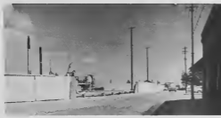
At a former blind corner west of WIMCO in San Nicolas, the Lago fence will be moved inwards (at the unfinished wall section) to provide better view to motorists of the oncoming traffic from the west and more walkway for pedestrians.
